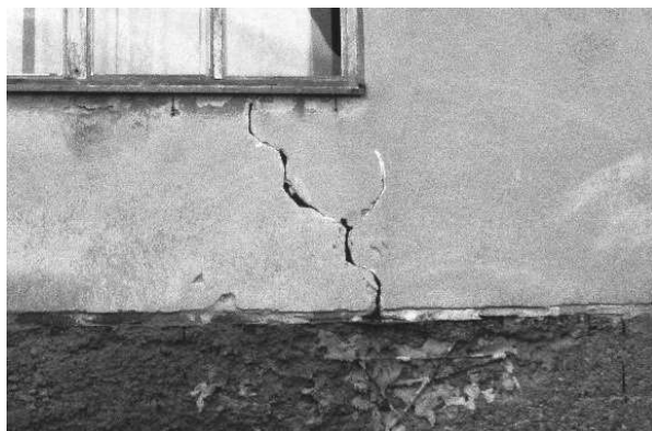
An example of the building structural defect
